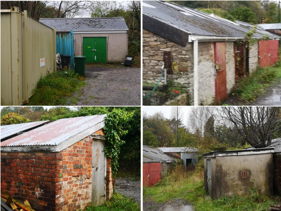
Mixed cluster of buildings – generally in a poor or very poor state of repair
